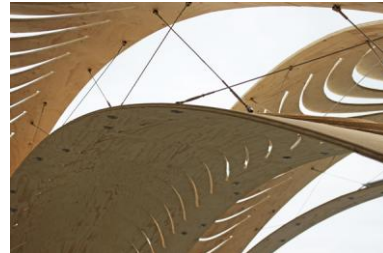
Figure 5. Detail of the sequence of stainless steel cables that stabilize the structure.
